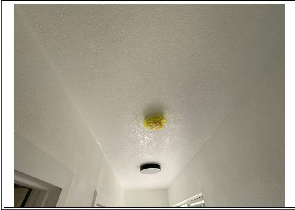
HALLWAY SMOKE DETECTOR
