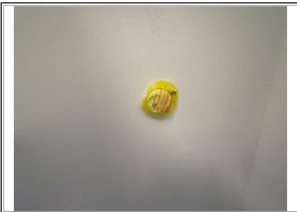
BEDROOM 2 SMOKE DETECTOR
