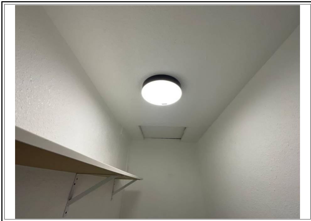
PANTRY LIGHT FIXTURES
