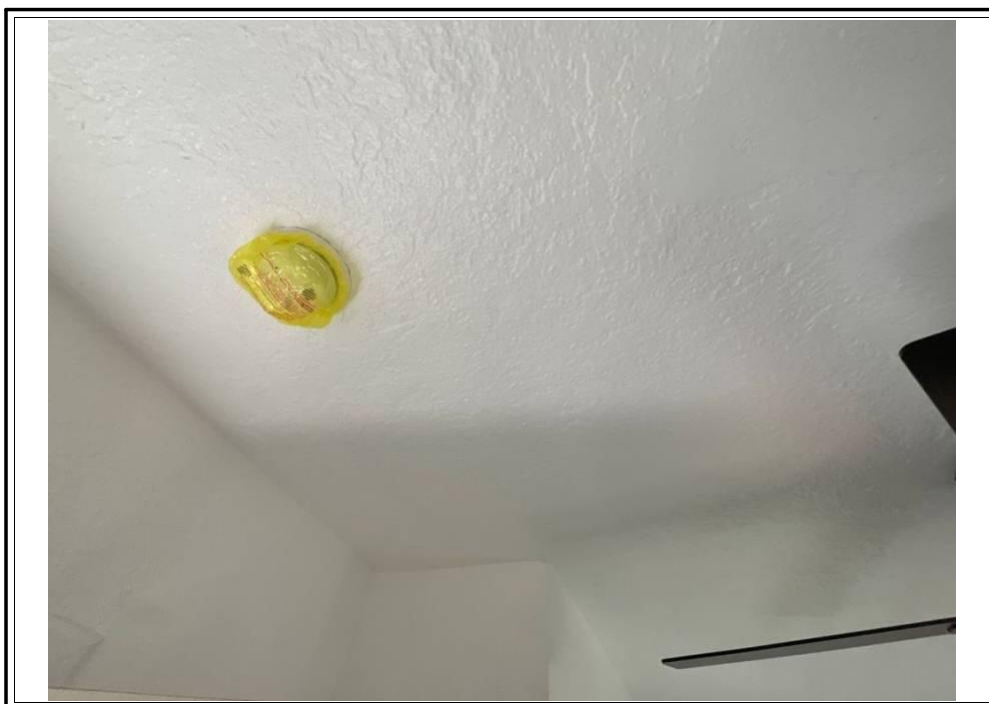
BEDROOM 1 SMOKE DETECTOR
