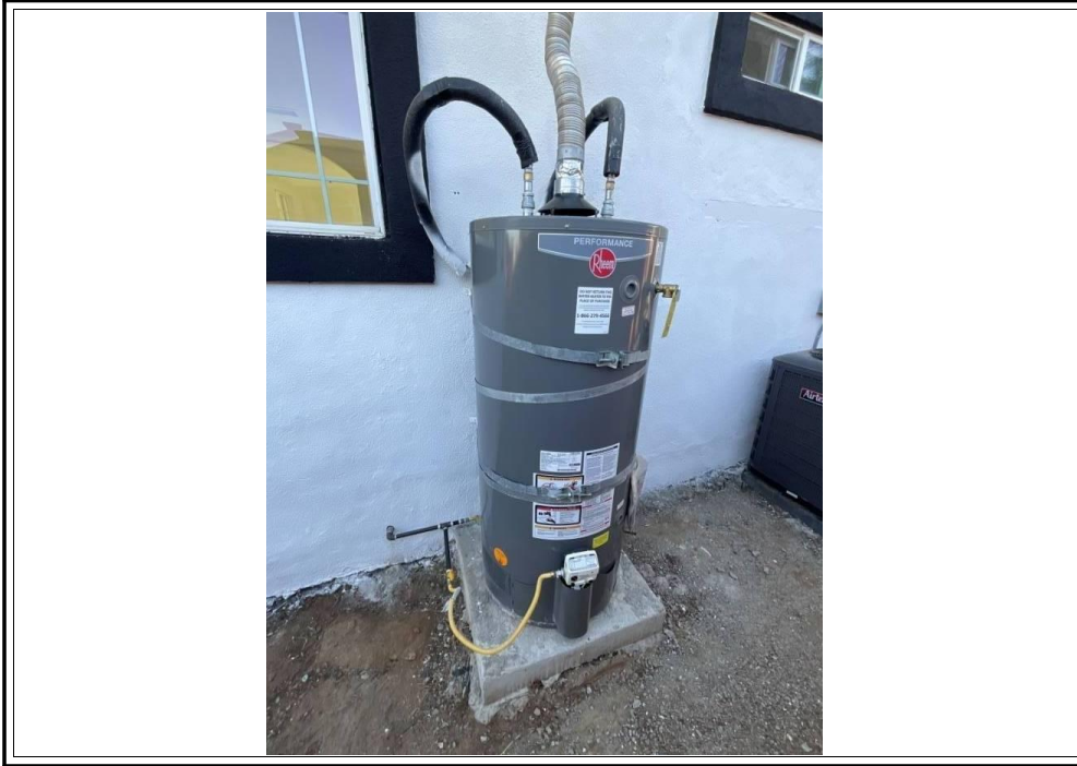
WATER HEATER - DOUBLE STRAPPED
